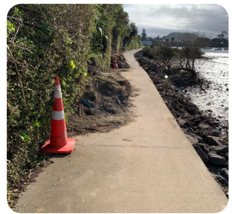
Image shows landslide three months later, after the gate closure had been removed. As you can see, there is no space for recumbent to pass.
