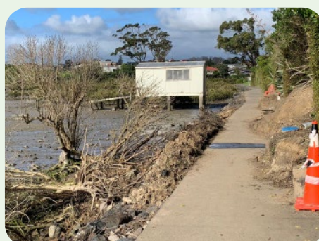
Landslip with no warning
