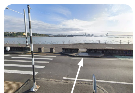
Sudden buffer on painted cycle lane, pushing cyclist out into traffic
